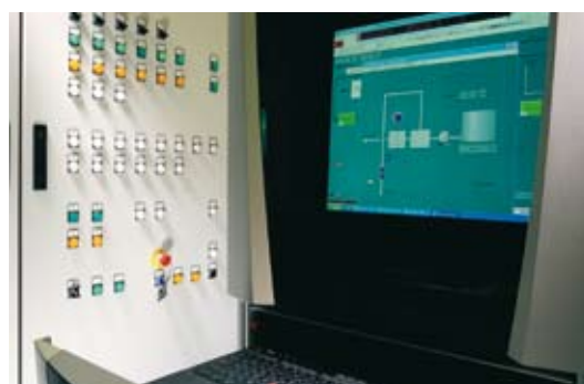
Remote monitoring of the BioBooster plant at Arla Foods in Hobro.
